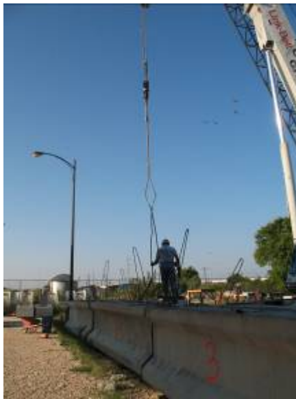
Figure D.12-3: Concrete beam being attached to crane with load cell to determine weight
