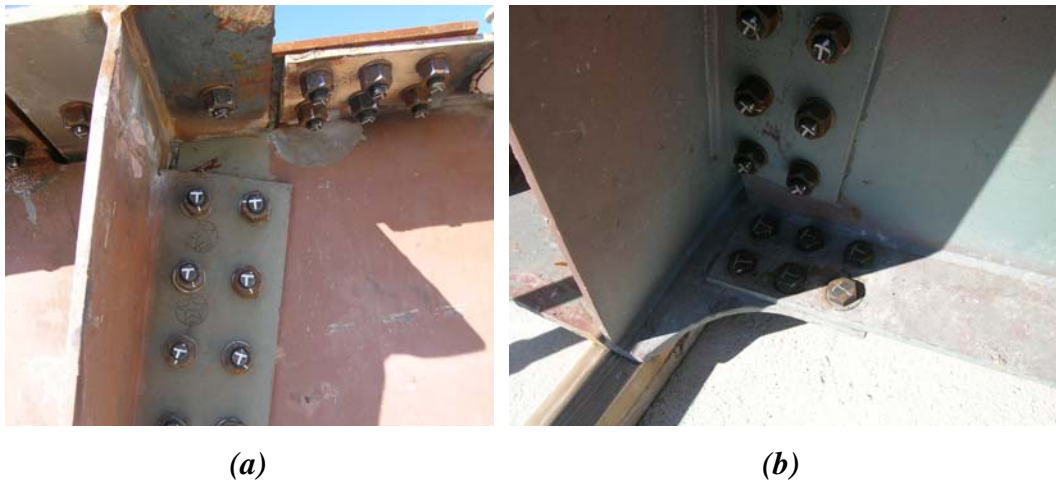
Figure 3.2: a) South end diaphragm top corner connection b) north end lower corner connection
