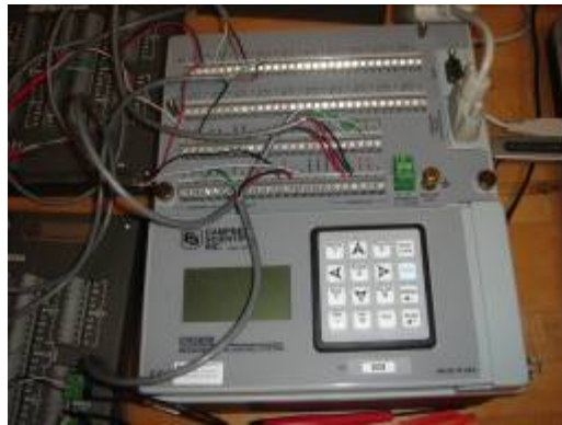
Figure D.11-3: Data logger unit used to collect data during construction phase of the project
