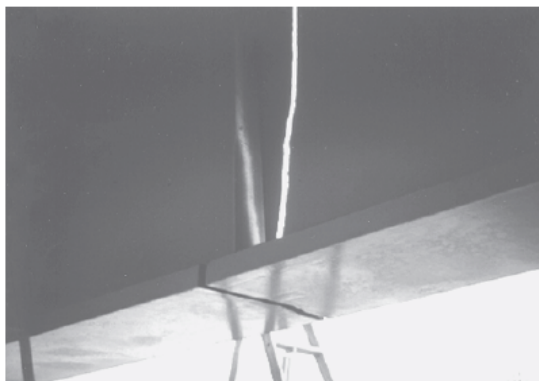
Figure 2.2: Girder fracture on a bridge on I-79 at Neville Island in Pittsburgh, Pennsylvania (Connor, Dexter, and Mahmoud, 2005).
