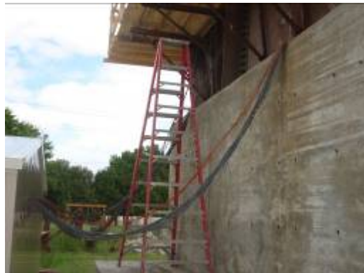
Figure D.11-1: Wiring coming from bridge to the data acquisition storage shed
