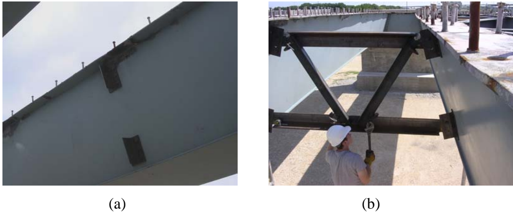
Figure 3.7: a) WT Stubs for external cross frames b) bracing being clamped together prior to welding.
