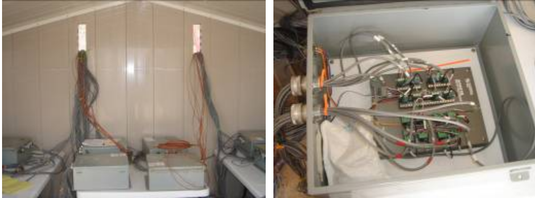
Figure D.11-2: Wiring routed to multiplexers and connected
