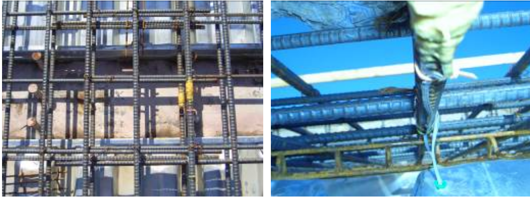
Figure D.8-1: Gages located in the center of the flange and the wires were routed under the bars for protection
