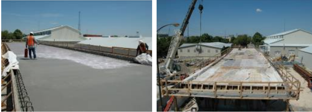
Figure D.9-3: Deck was sprayed with sealing compound and covered with wet blankets and plastic to cure
