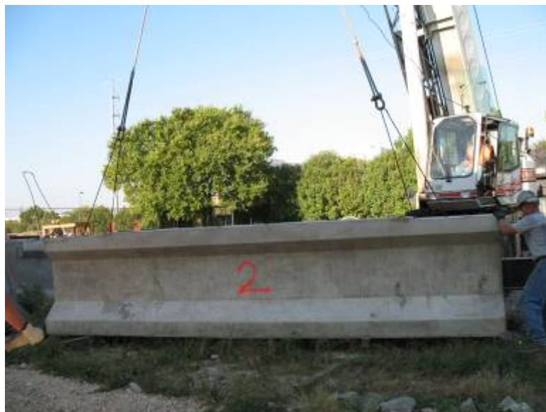
Figure D.12-4: Beams were numbered to keep track of strain from load cell and position on the bridge deck during testing
