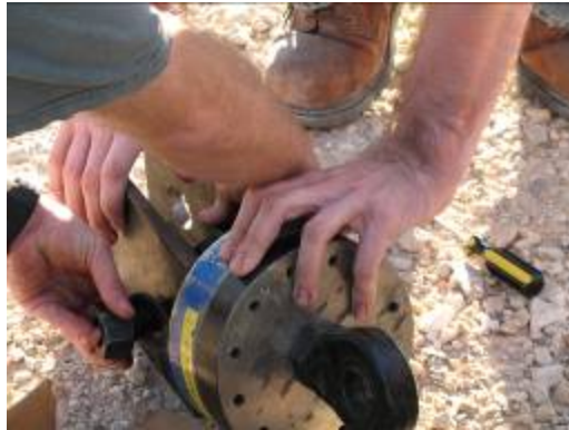
Figure D.12-1: Attaching plates to load cell to allow it to be hooked to crane cable
